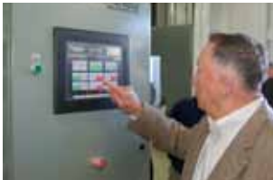
Viking president and co-founder Bill Healey demonstrates the custom touch-screen control panel, which flows electricity and hot water throughout the building.
